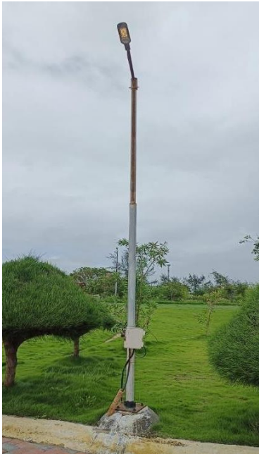
Parking area pole
