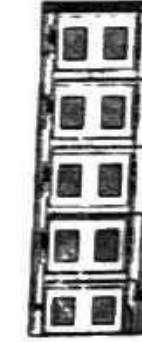
Marshalling Rack 2CVA01 2 Cubicles
