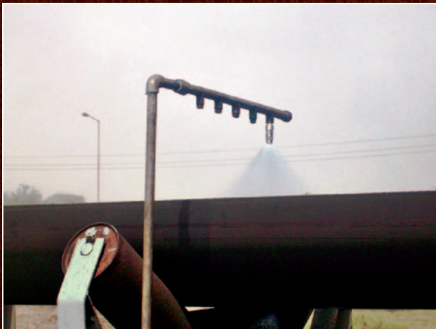
Dry fog system for lignite conveyor
