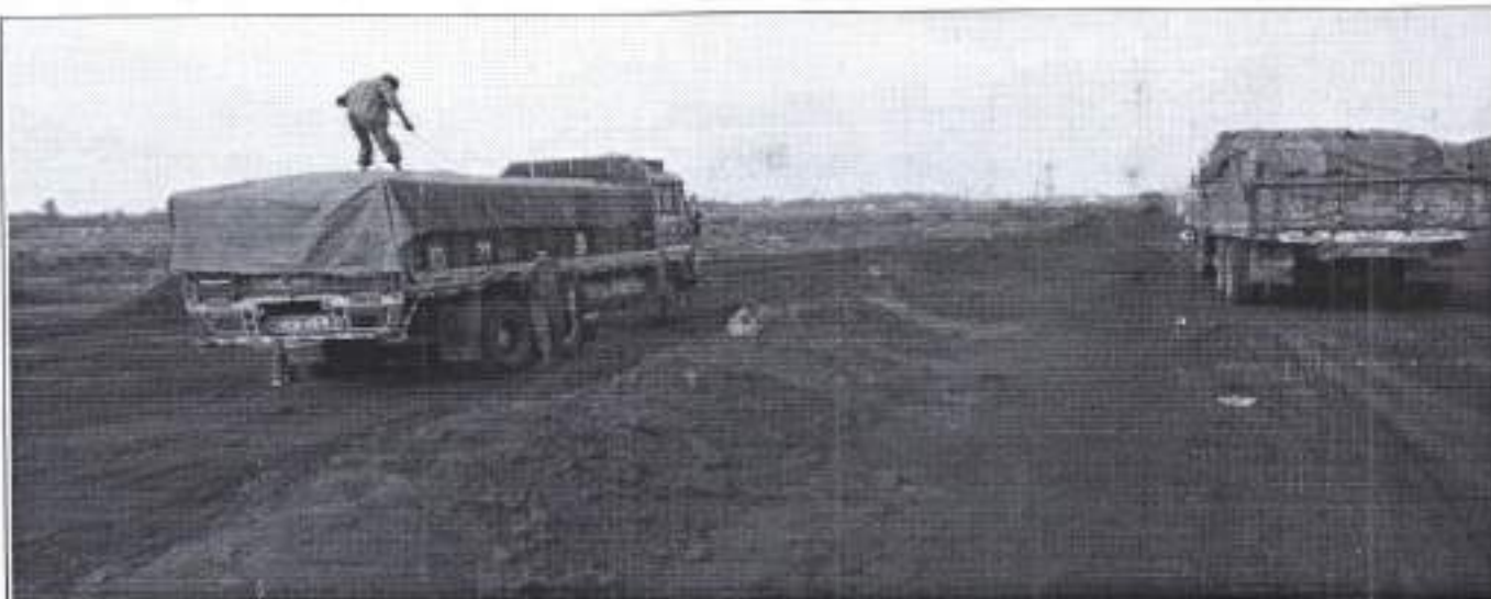
Covering with Tarpaulin of Loaded Trucks
