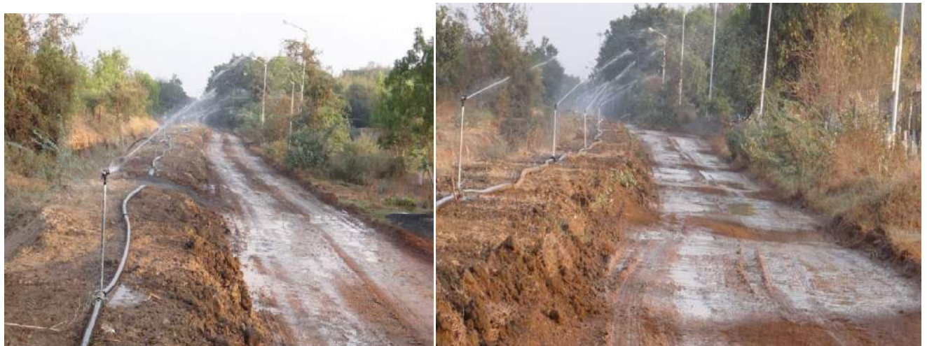
Continuous water sprinkling system for dust suppression
